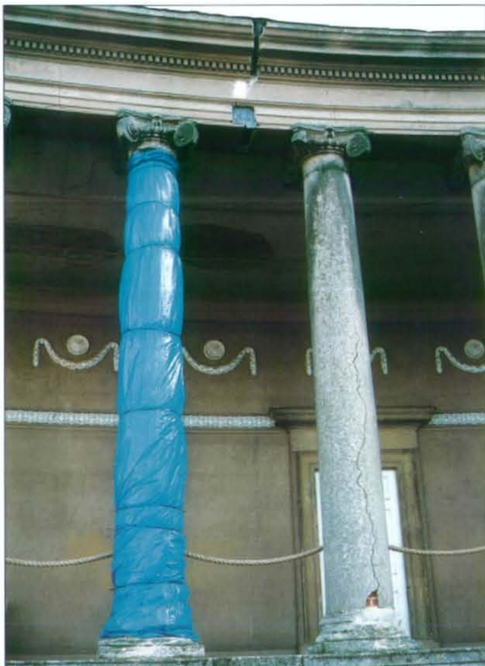
Preparatory work had removed the stucco from a column, revealing the brick beneath. It was later protected from the weather by the brightest of blue plastic coverings.
