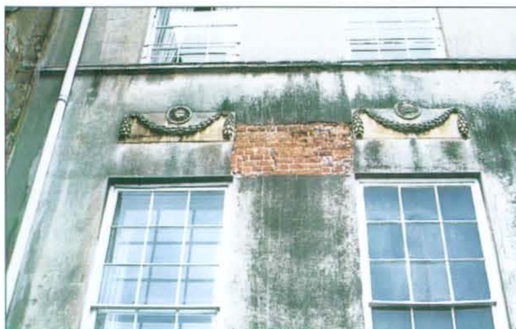
Stone slabs above ground floor windows of the central pavilion with decorative festoons and paterae. Exploratory work has revealed some brick beneath the stucco.
