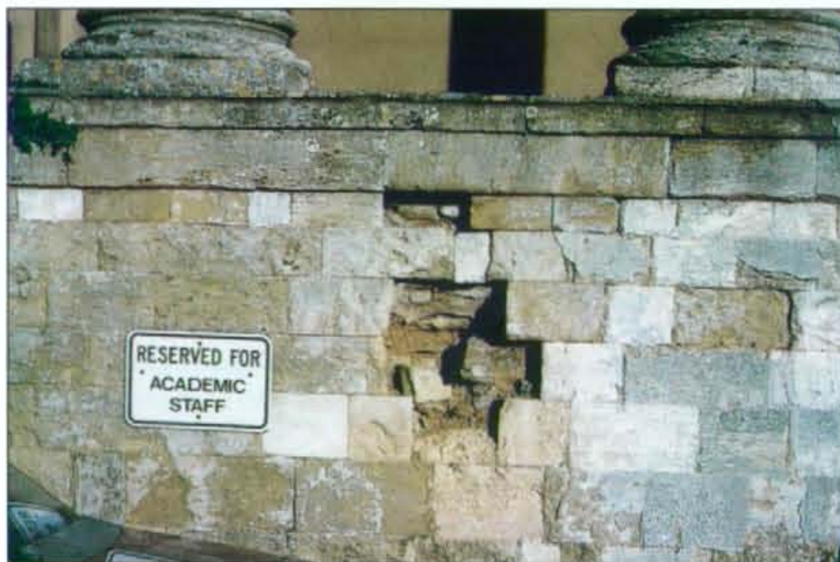
The facing of ashlar on the podium of the Grenville colonnade. Clearly some sections of ashlar have been replaced in the past. Exploratory work shows messy rubble behind the smart dressed stone. Above are two worn stone bases of columns.
