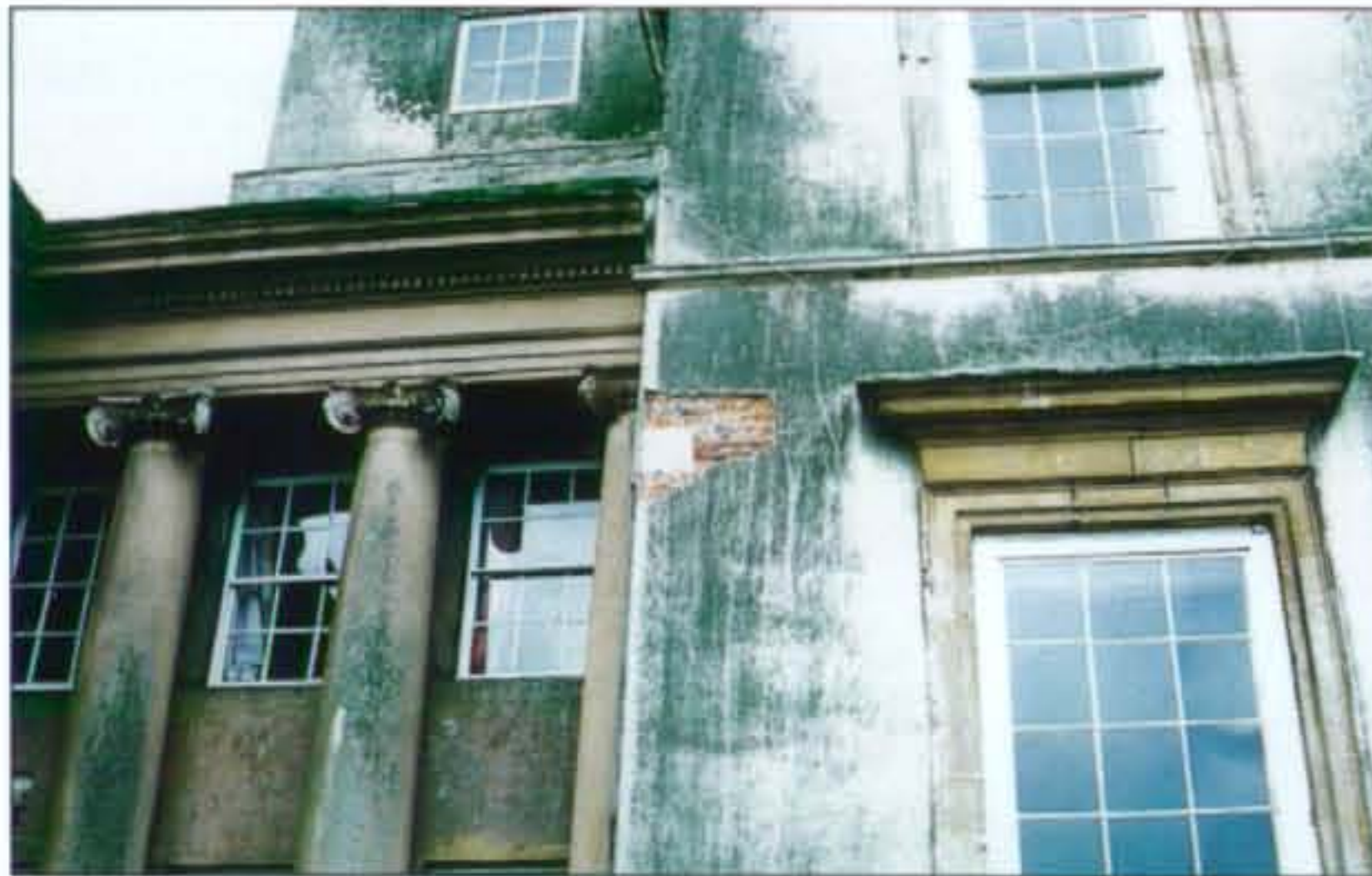
The dirty stucco has been taken off on one section to reveal beneath red bricks and a white decorative quoin, part of the original mansion of the 1670s.
