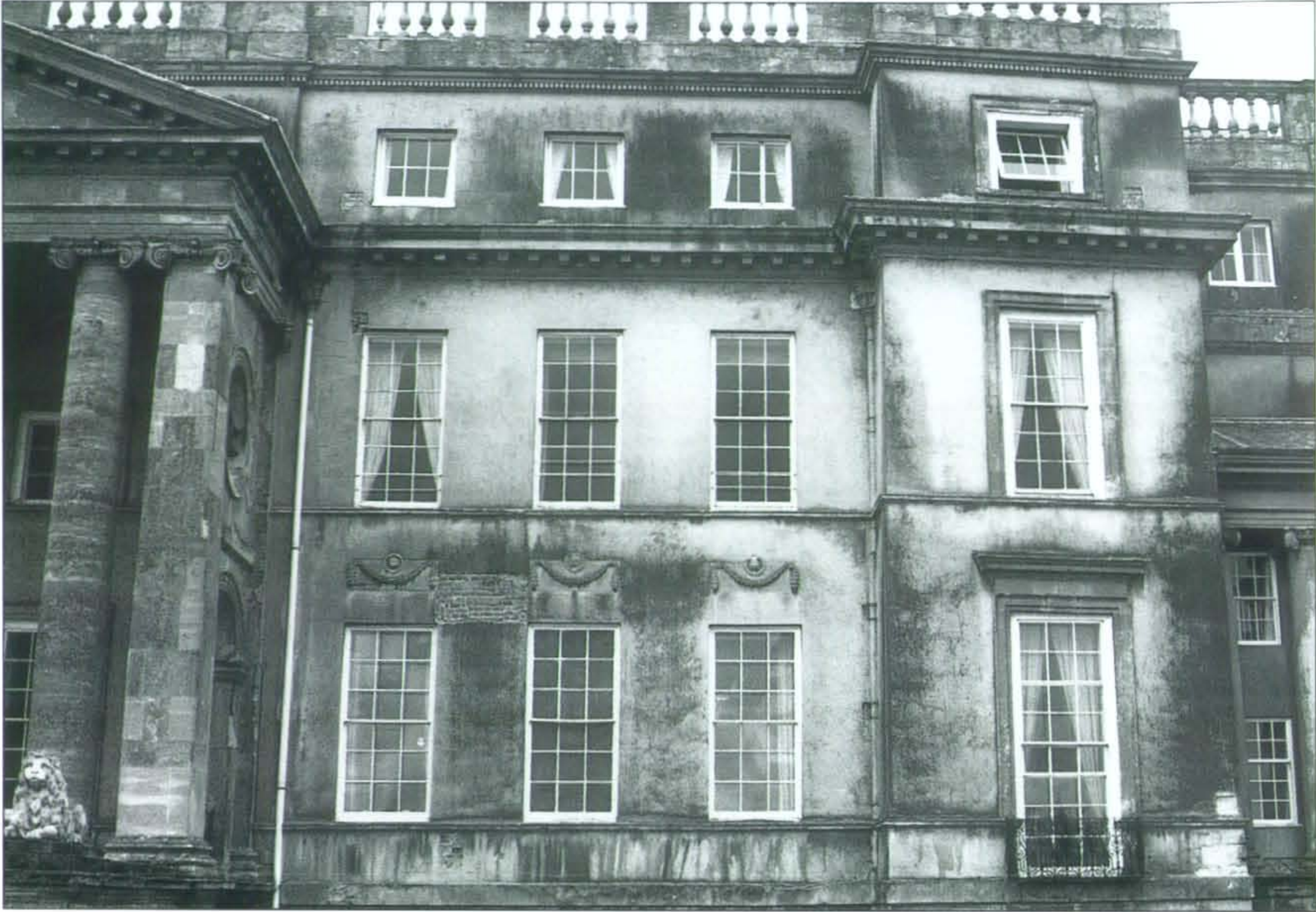
December 1999: Exploratory work has chipped away the stucco in several places to reveal the original red brick
