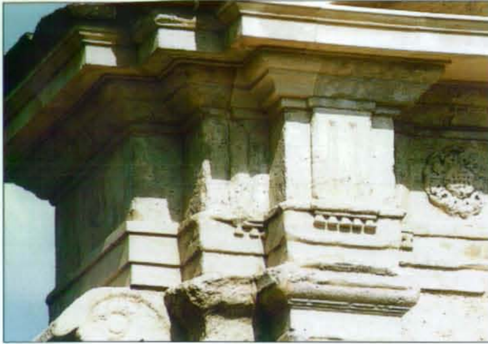
New stones are very clear in this close-up of one of the restored Leoni arches. An indication of the kind of restoration work to be carried out on other stonework on the North Front.
